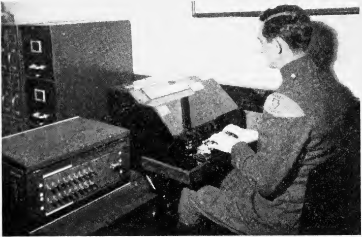
Switchboard and associated teletypewriter: Harrisburg installation, Pennsylvania State Police teletype network.
